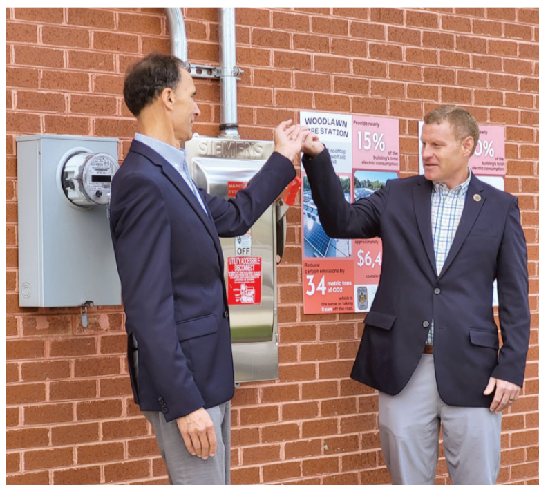
Chairman Jeff McKay and Supervisor Dan Storck flip the switch to turn on the solar panels.
